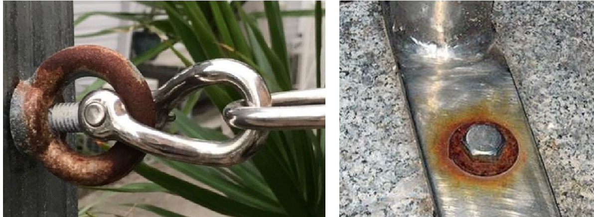
Fig. 7. Two examples of contact corrosion at atmospheric conditions between stainless steel and galvanized plain steel
